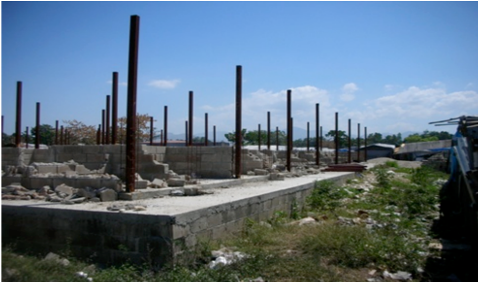
Figure 1 Central Market, Leogane, Haiti. Two years after 2010 earthquake.
